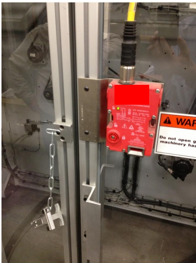
Category 4 rated switch not applied per manufacturer’s requirements or relevant standards, and thus subject to a single point of failure due to mechanical application issues, i.e., chain (breakage) or fastener (single button head screw barely larger than the chain link).
